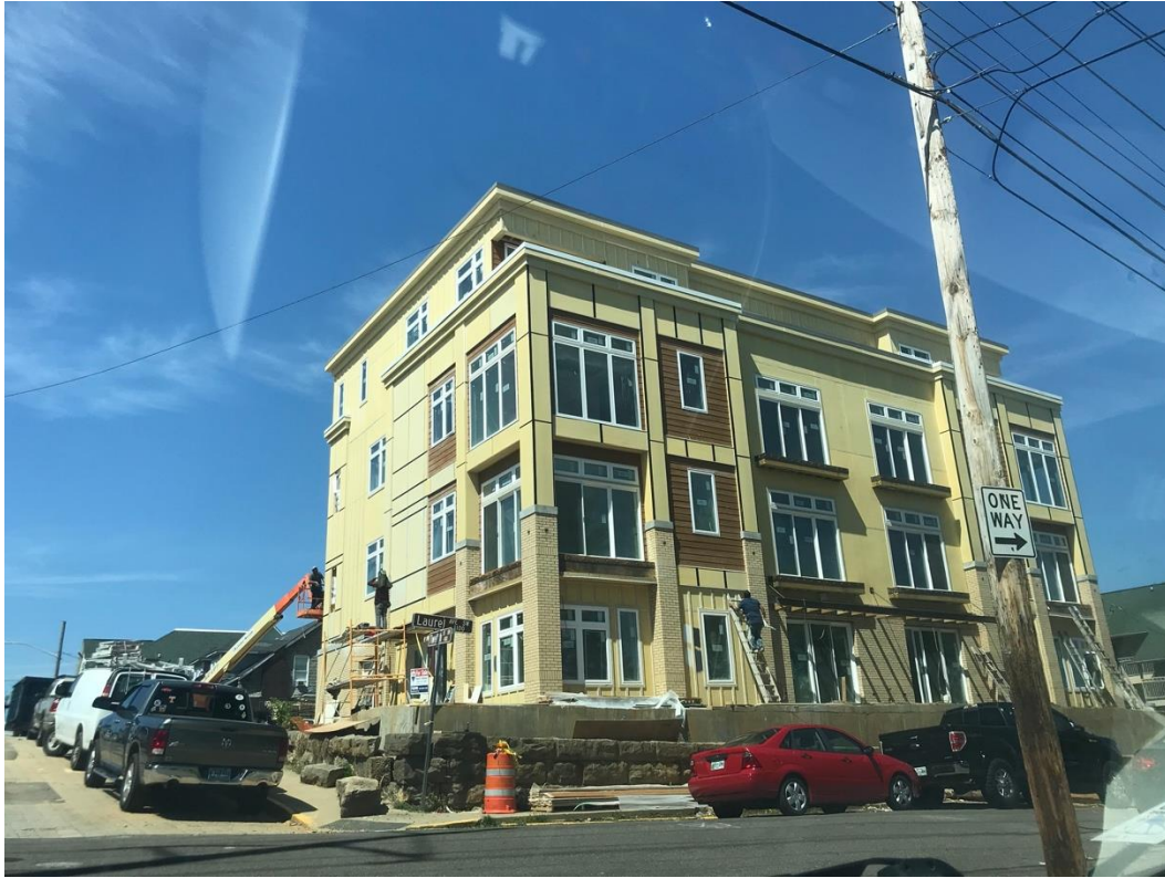
Figure 4: New luxury student apartment development being built in the Fort Sanders neighborhood. Source: Yael Uziel
